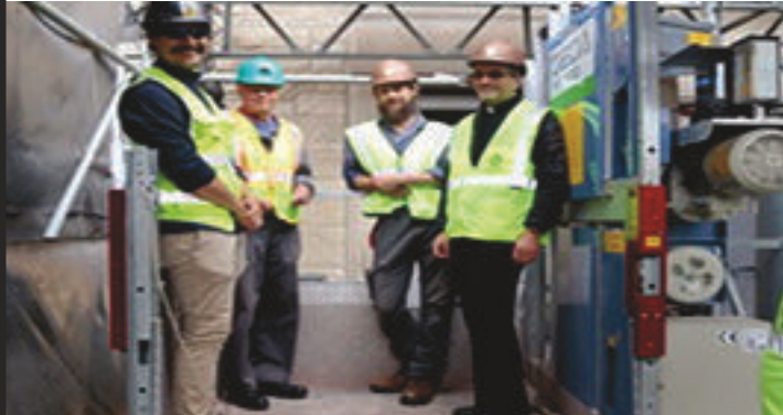
Jamieson Mar-Pohl, Bob Perlock, Nathanael Rhody, and Msgr. Gilles in the GEDA hoist ready to inspect steeple damage. In the upper right, you will see a large slab of stone which has let loose.
